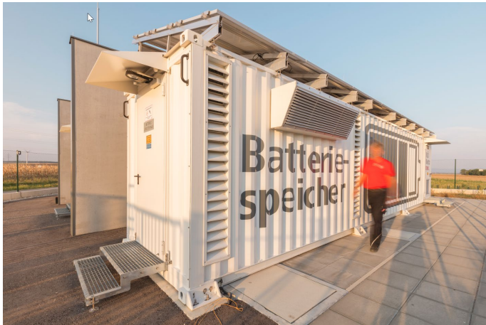
Utility-scale battery storage
