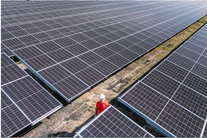
Large-scale PV plant
