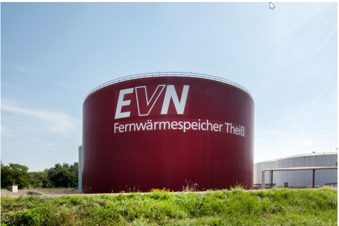
Hot water storage
